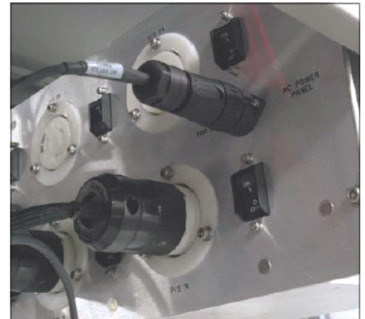
AC Distribution Box
